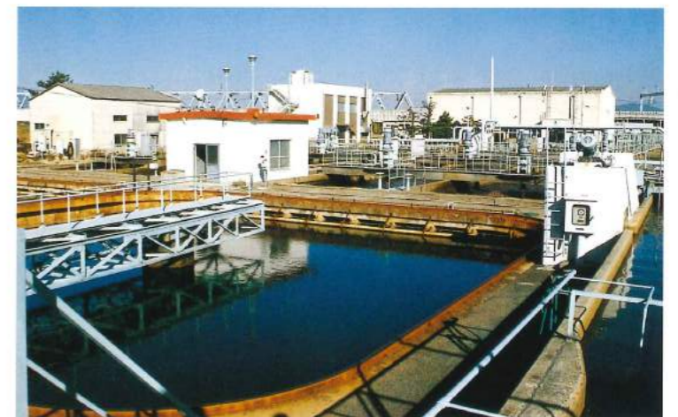
12 The Noda Drainage Plant, which began operations in 1935, still in operation today with the original pump house, first and final pools for floating matter deposits, and clarifier.
