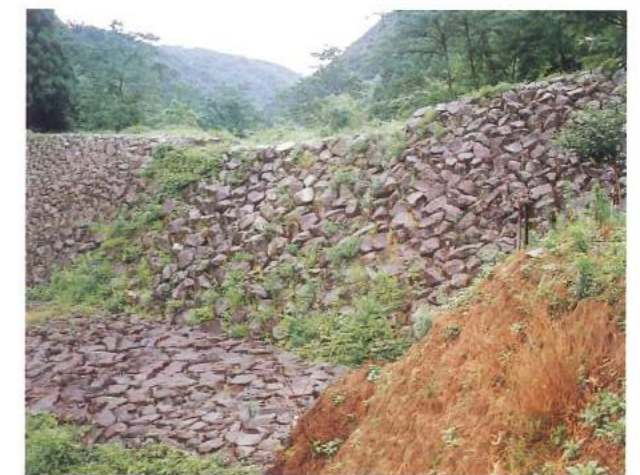
81 The Hanedani Dike, constructed in 1888, is composed of huge stones and serves to prevent rock erosion in times of heavy rainfall. It is 12 meters high and 54 meters wide, the largest of its kind for its time.
