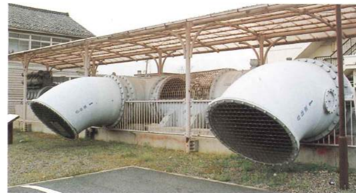
83 The old vertical-axis Umori drain pumps, built in 1936, were in operation for 40 years. They were run by diesel engine (300 hp), and water drainage output was 3.25 cubic meters per second.
