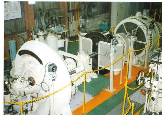
34 The First Miyashiro Power Station, built in 1904, is the oldest working power station today. It utilizes a century-old German water wheel and generator.
