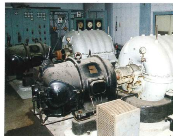
11 The turbo-blower and motor used in the revolutionary Japanese process called the activated sludge method, housed in Horidome Drainage Plant which began operations in 1930.
