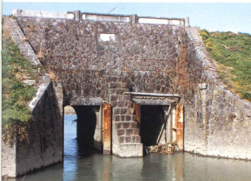
71 The Goroku Sluiceway, built in 1907. It is composed of two arches and steel doors that closed automatically when the water level at the downstream region became higher than that on the other side of the doors.
